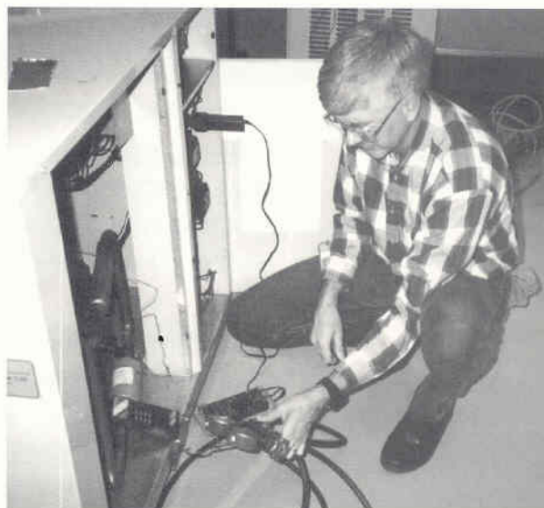
Checking system superheat at the condensing unit.
