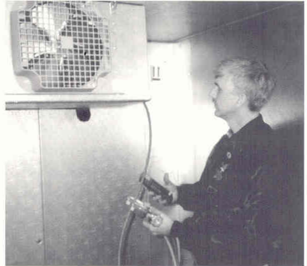
Superheat should be adjusted at the evaporator expansion valve.
